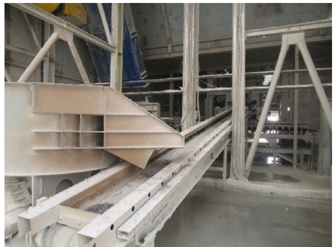
Fibre Dosing Unit with buffer conveyor belt
