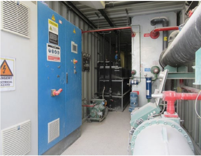
One of the Chiller Units
