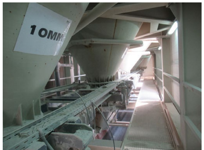
Level 2 in Building 2, showing the material silos
